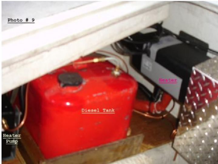
Photo 9. Diesel tank and heater in the port compartment.
