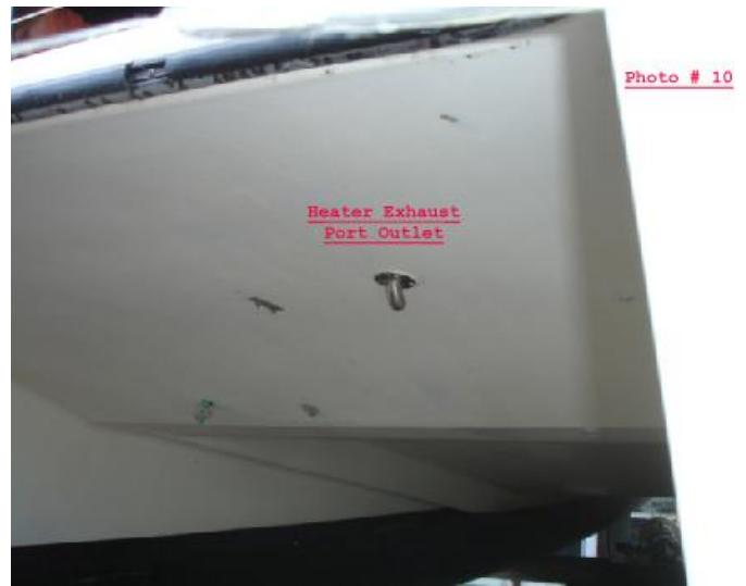
Photo 10. The heater exhaust exiting the forward hull.
