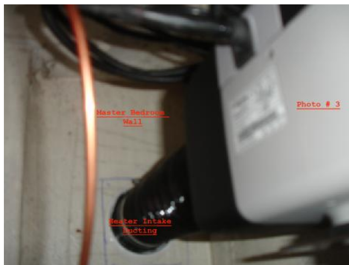
Photo 3. The duct exiting the heater and into the master bedroom wall.
