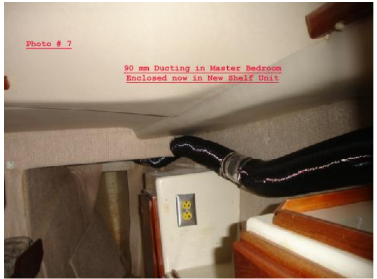
Photo 7. The 90 mm ducting in the master stateroom. It is now hidden within a new shelf.
