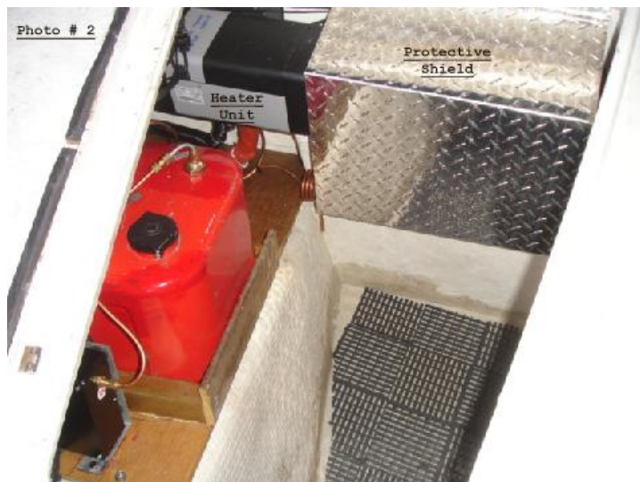
Photo 2. The heater is mounted on the bulkhead wall between the head and the port sail locker. A protective shield ...
