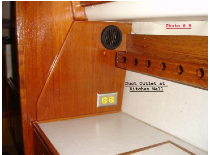
Photo 8. The duct outlet at the kitchen wall.
